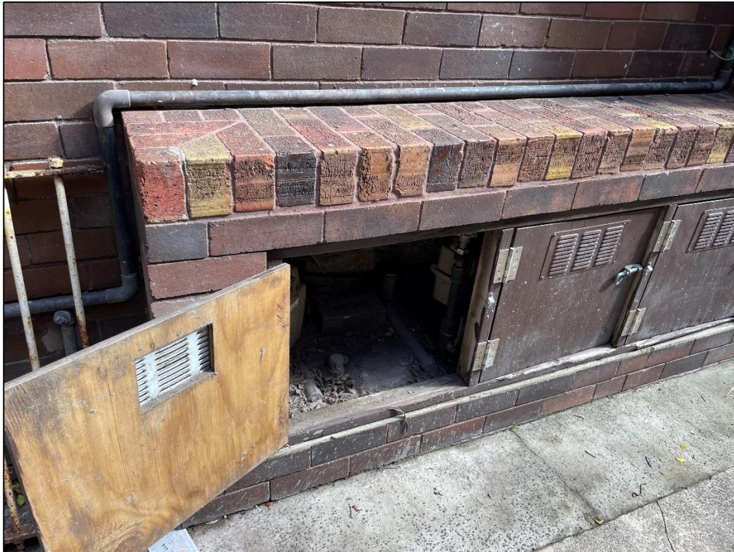
Photograph 1 Location of 'Monitor 1', affixed to the brick façade (within the gas meter enclosure) on the northern side of the building, approximately 15 m from the closest edge of works.
