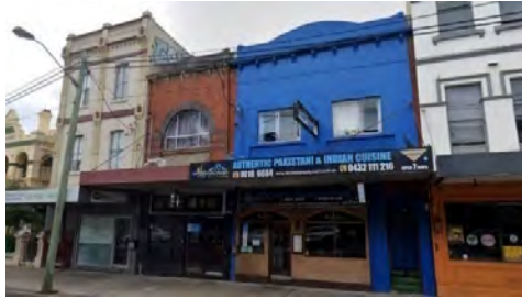
Figure 28: Inappropriate paint finishes
