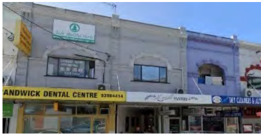
Figure 29: Inappropriate infill window / glazing framing
